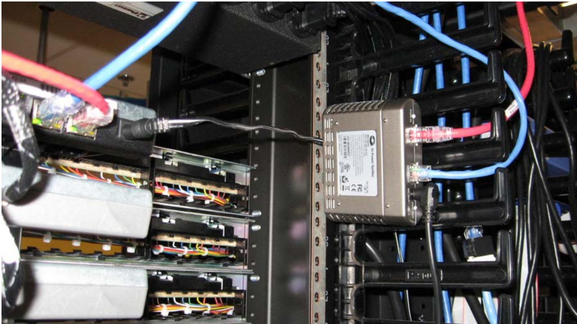
Figure e) PoE splitter mounted near Panel Manager
