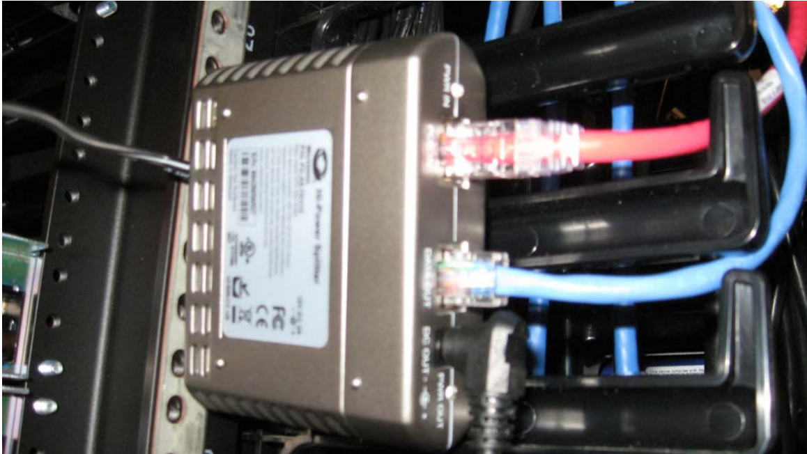
Figure d) PoE mounted behind the rack
