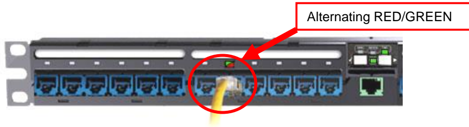
Figure 42 - Patch Panel in Trace Mode
