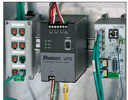
Figure 4. The Panduit Industrial Network UPS with ultracapacitors remotely displays the health of two power supplies, the UPS and temperature.
