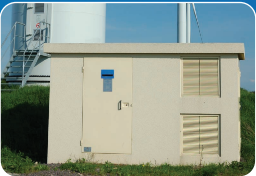
Substation and Control Room
