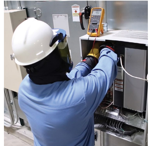
Figure 1. Absence of voltage test using a hand-held voltage test instrument.
