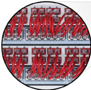
Direct Switch Patching with 8 inch Patch Cords
