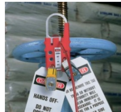
Figure 9. Equipment being locked out using Panduit Multiple Lockout Device PSL-MLD, which can be used alone as a lockout hasp, or with the provided cable to lockout electrical disconnects, gate valves, or large cumbersome devices.
