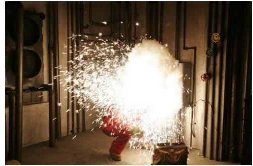
Figure 2. An arc flash event on an electrical panel in an industrial facility.
